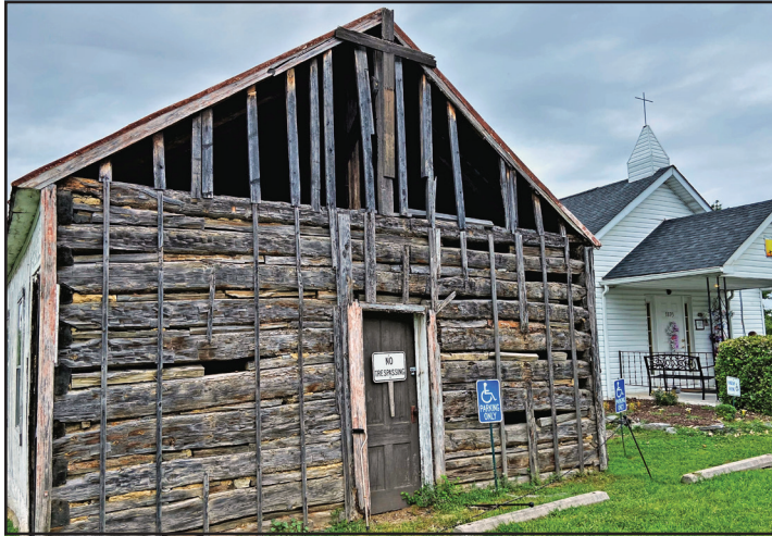
In 2022, the front of the historic Log Cabin Church in Middletown, estimated to be the oldest building in the town, built between 1816 and 1819, showed the considerable wear it sustained over the years.
