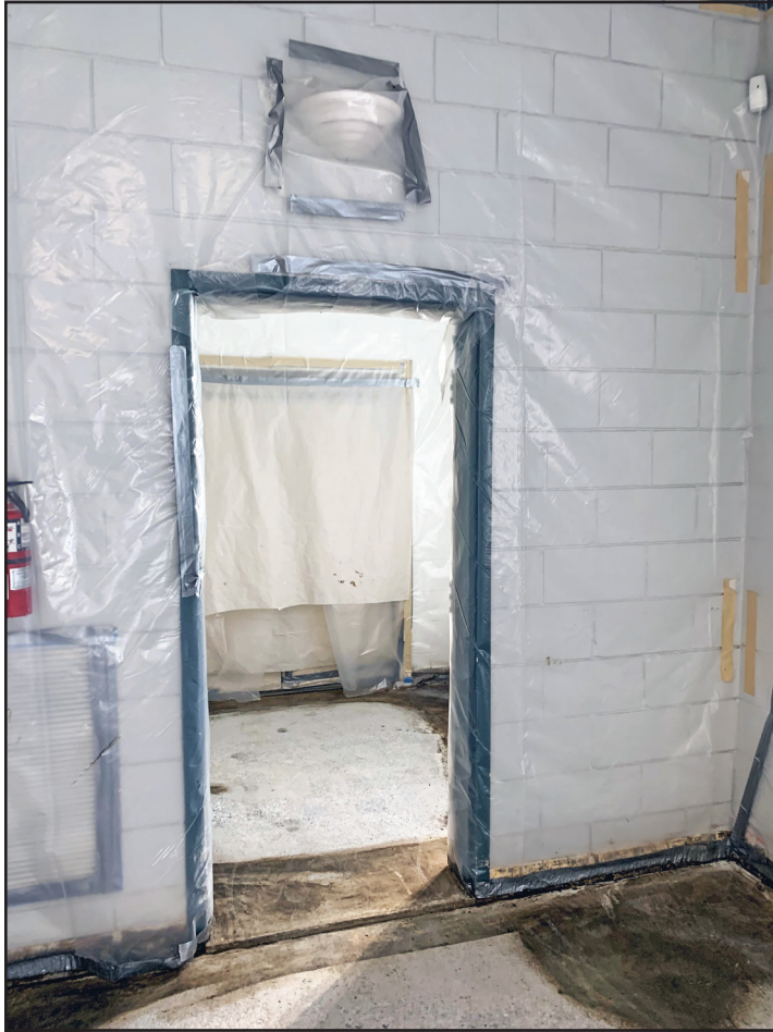
Here is an example of one of the “before” areas inside the former Raymond E. Santmyers Youth Center at 200 E 8th Street. Extensive repairs and renovations have been done to ready it for use as a new clean, safe place for the Warren County youth to meet.
